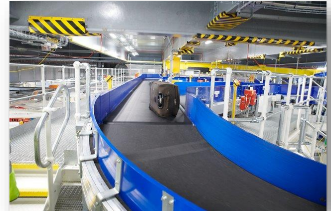
Baggage screening area to be upgraded to the latest generation equipment
